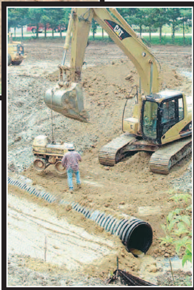
(Above and Right) Sitework begins on Greatrex Place in the Summer of 2004.
